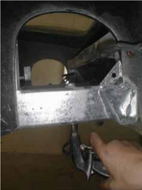
Blow out threads & pin holes
